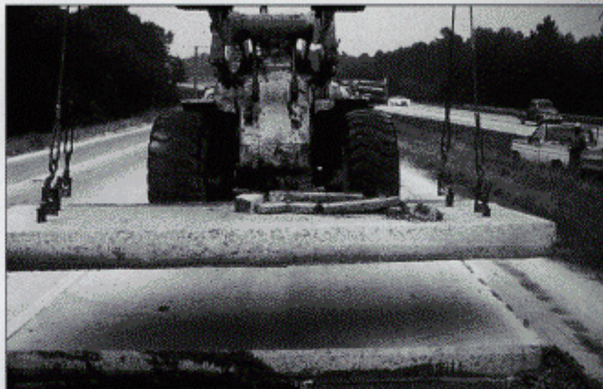
Figure 1. Whenever possible, lift deteriorated concrete out of place rather than breaking it. Lifting the old concrete imparts no damage to the subbase and usually is faster and requires less labor than breaking the concrete before removal.
