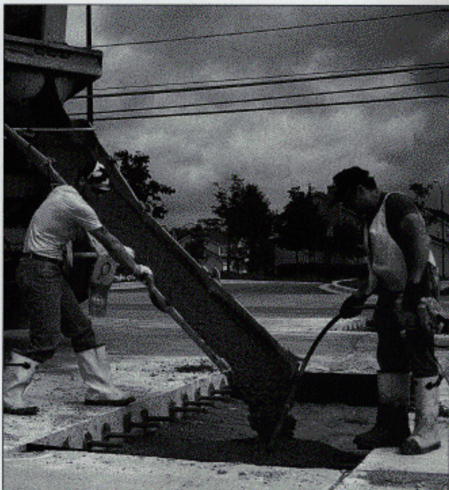
The methods used to remove old concrete, install dowels, and place and cure the repair concrete can greatly affect total repair time.
