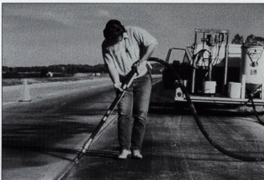
Reservoir preparation is the most important step of a joint resealing project. Above, a worker sandblasts the top of a joint face to provide a clean bonding surface for the sealant.
